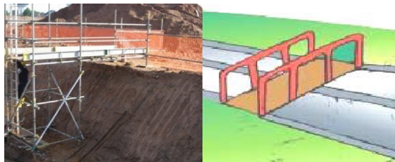
Safe Access Platforms
